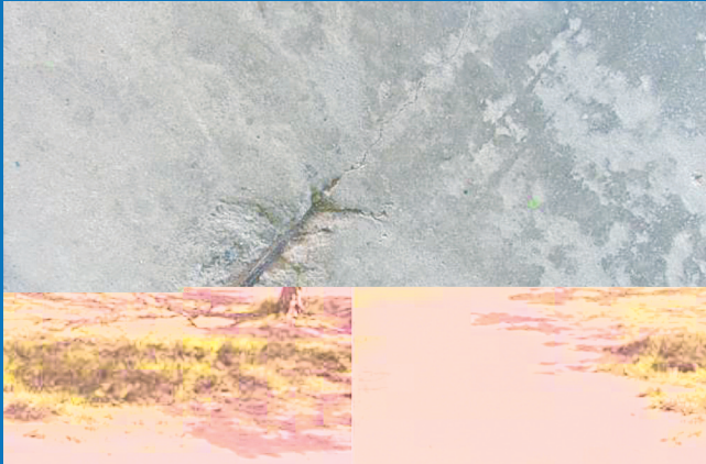
■ FLOOR SLAB TO BE REPAIRED
