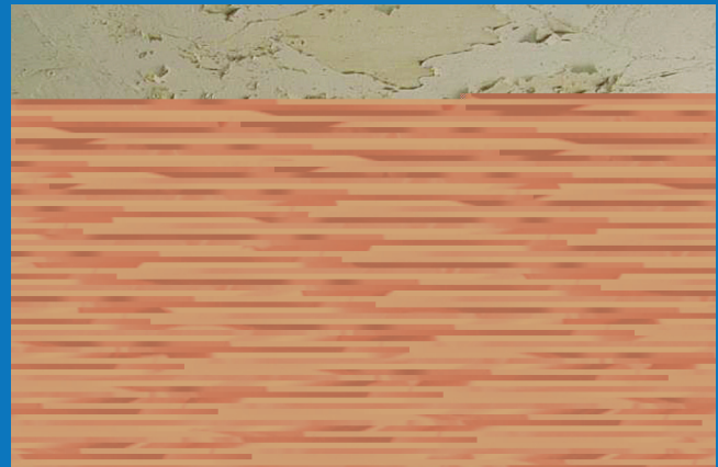
■ PEELING PAINT – INDICATIVE OF MOISTURE PENETRATION
