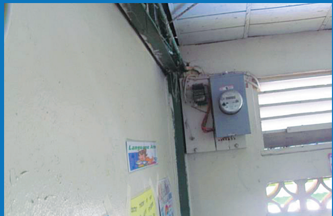
■ ELECTRICAL PANEL IN CLASSROOM
