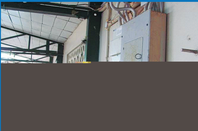
■ ELECTRICAL PANEL IN CLASSROOM
