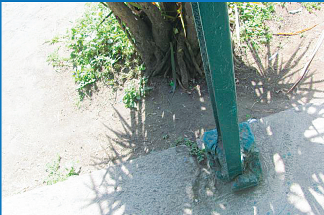
■ STANCHION SUPPORTS IN NEED OF REPAIRS
