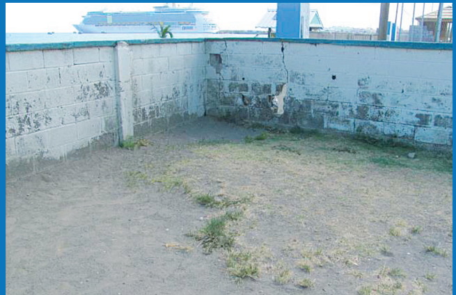
■ FENCE WALL IN A STATE OF DISREPAIR
