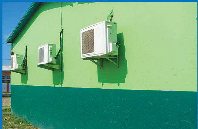
■ A/C UNITS INSTALLED FOR SPECIALISED ROOM
