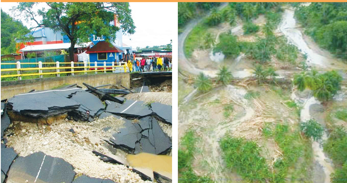
FIGURE 3.1: IMPACTS OF HURRICANE TOMAS (2010). SOURCE: SLU DRR
