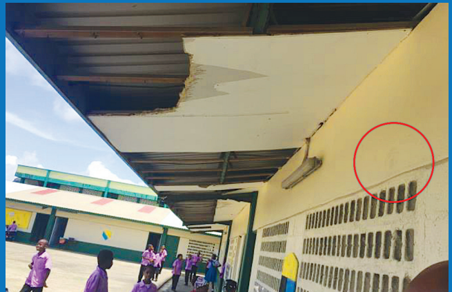
■ WATER DAMAGED CEILING
