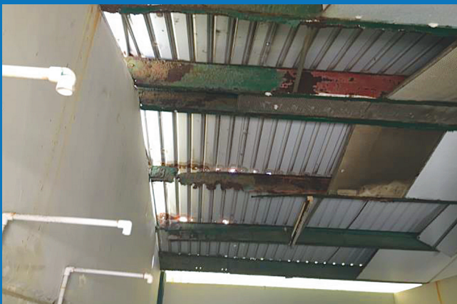
■ CORRODED ROOF STRUCTURE OF TOILETS
