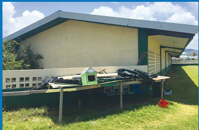
■ TYPICAL END VIEW WITH EXCESSIVE EAVES
