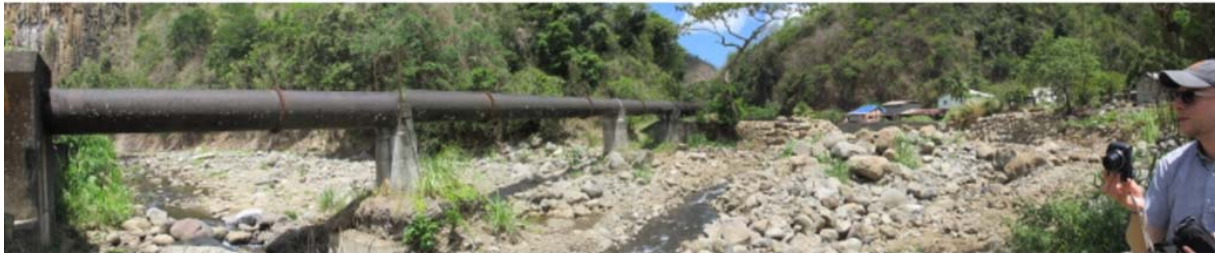
Figure 4-12: Damage due to Christmas eve 2013 rainfall event. .
