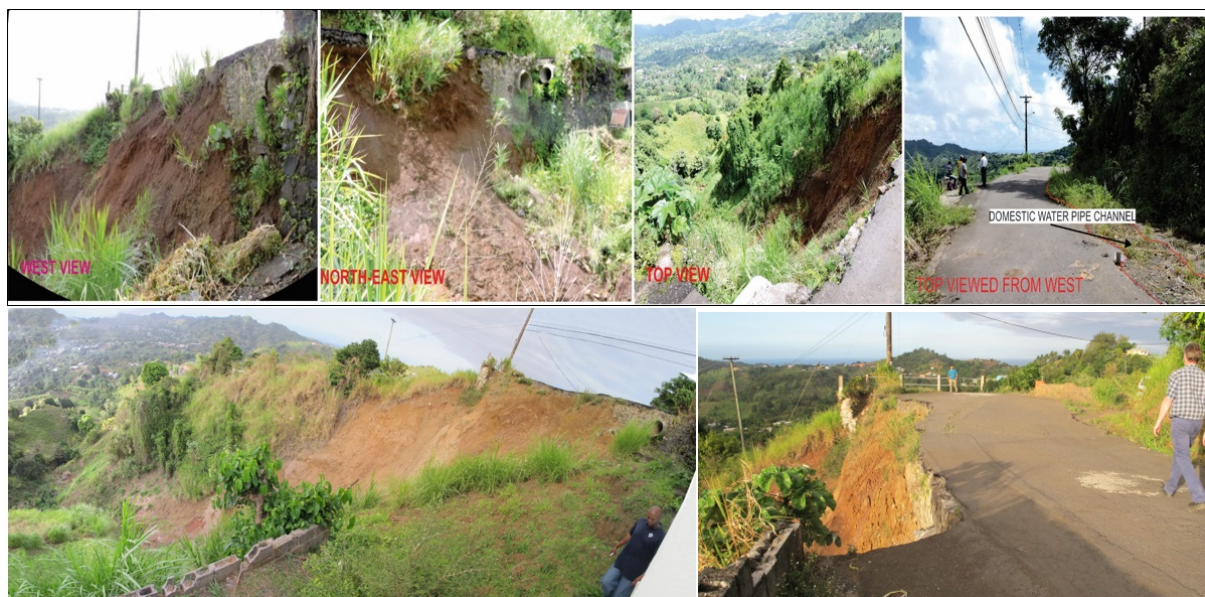
Figure 4-4: The Belmont landslide.
