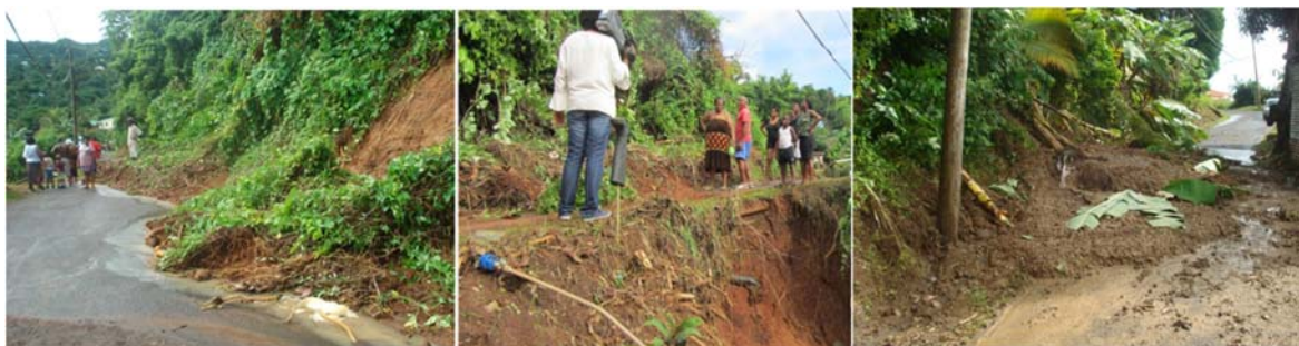
Figure 4-9: Small landslides affected the road network that occurred in Morne Delice in January 2011.
