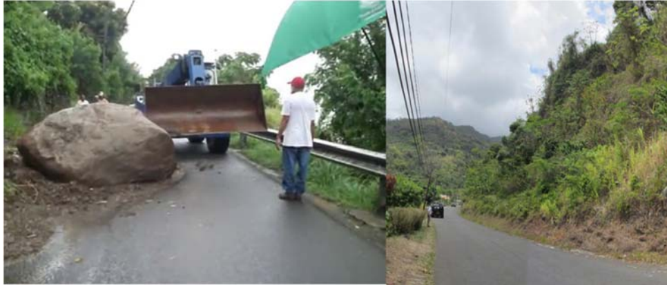
Figure 4-7: Rock fall problems around the coastal road from St. George's to the North. Left: Rock fall in Maran St. John's in April 2011; Right: location of rock fall tragedy claiming 9 lives of persons in a bus that was hit by a rock in the village of Cotton Bailey in 1991.
